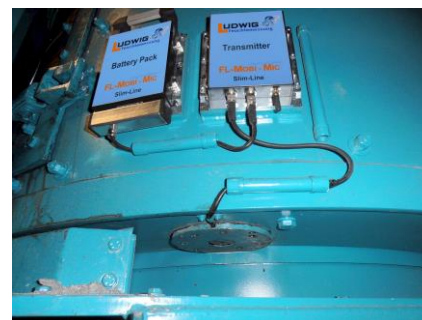
Installation of probe, transmitter and Akku pack at a mixer with rotating drum
